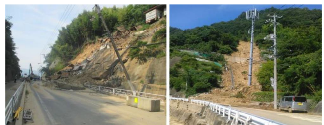
Photo 7 Retaining wall collapse (Fig.11, No.1) and slope failure (Fig.11, No.2) made the Hiro-Nagahama an island on land
